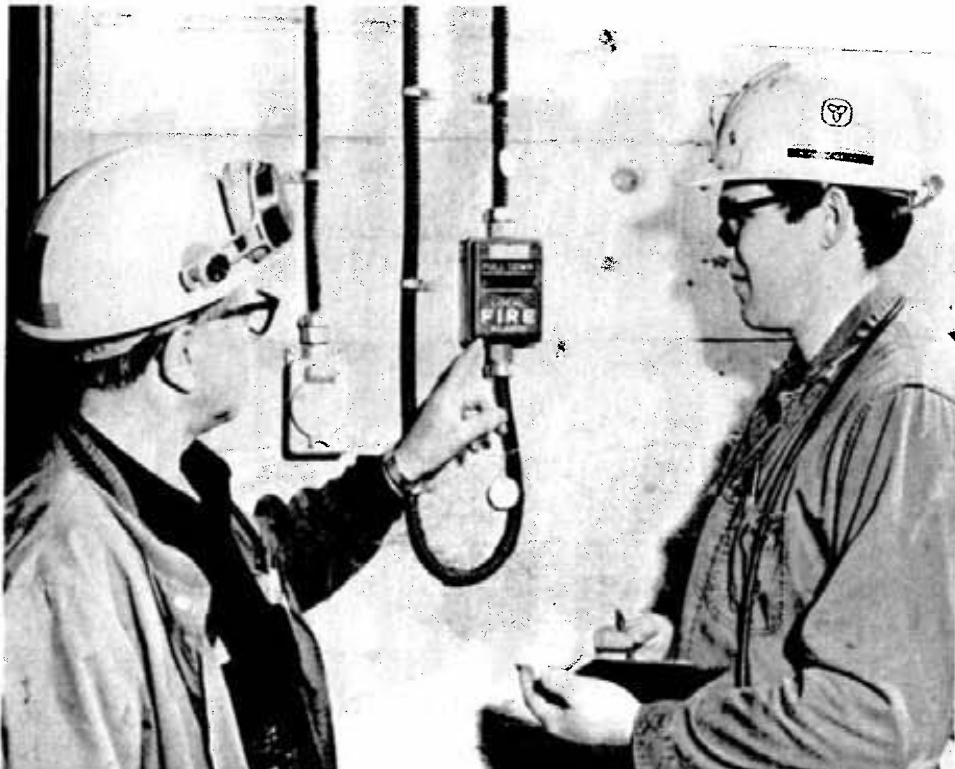
Inspecting one of the two manual "pulls" that will also activate the new fire suppression system are Ken Stone, left, Froid-Stobie safety supervisor, and Michael Reiser, electrical mechanical engineer, Ministry of Labor.
