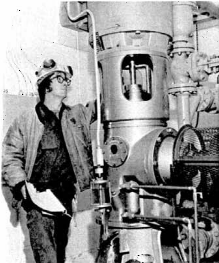
The pumps and motors that provide fresh water to the mine's underground and surface operations are inspected weekly to ensure continuous operation.
