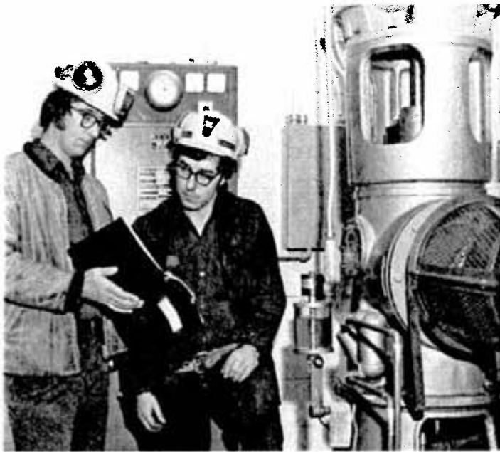
Electrical foreman Art Robinson, left, explains the operation of the Garson mine number two deep-well pump and motors to first class electrician Cleo Roy.
